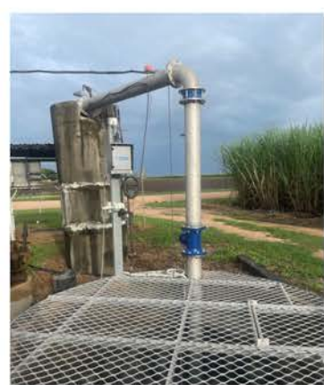
Live flow and nitrate sensor mod on centrifical pump
